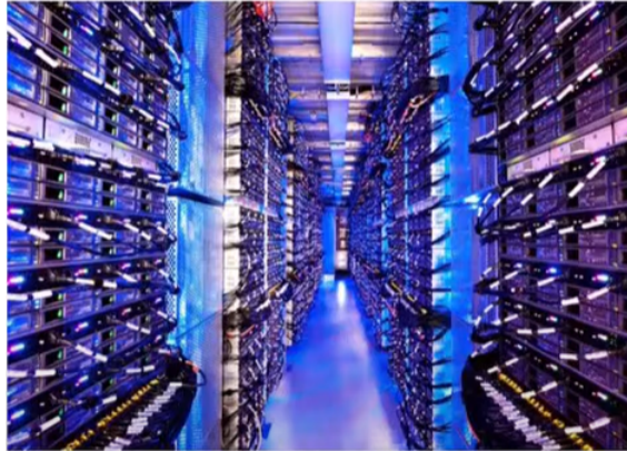
Figure 11.4: An aisle of a data center
